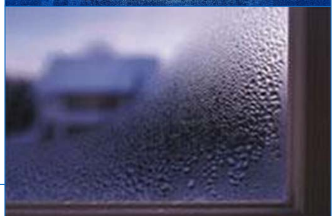
Condensation on the inside of a windowpane.
